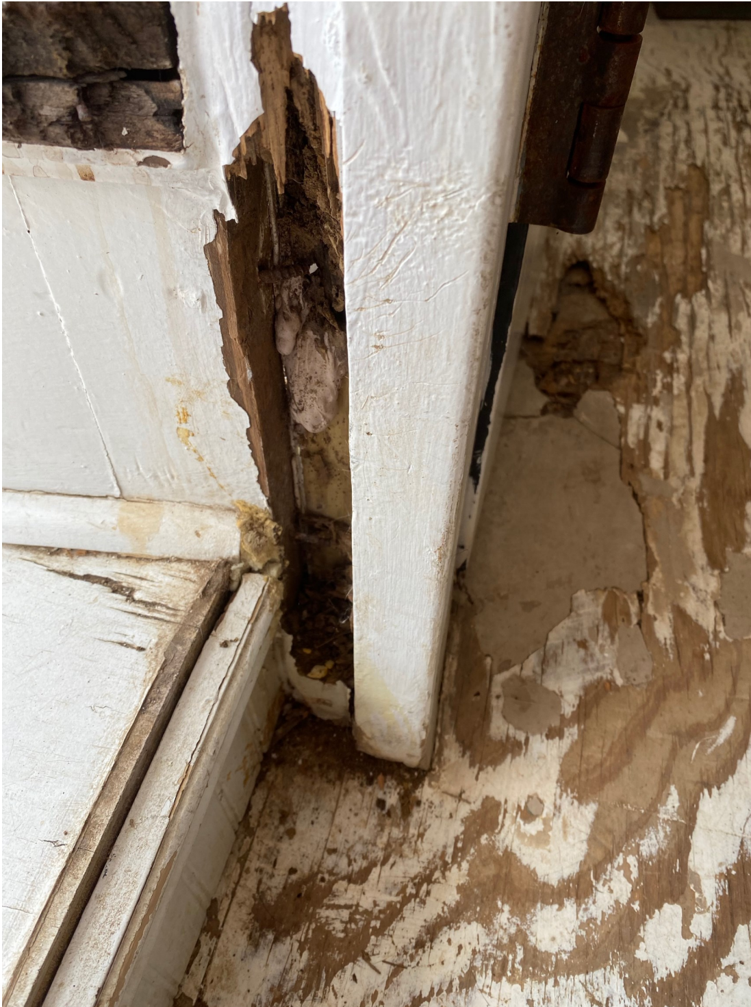
Door Frame Damage
