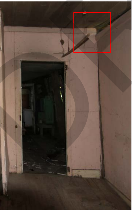
Displaced Wall in Back Bedroom
