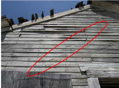
Nails from Porch Roof on East Elevation
