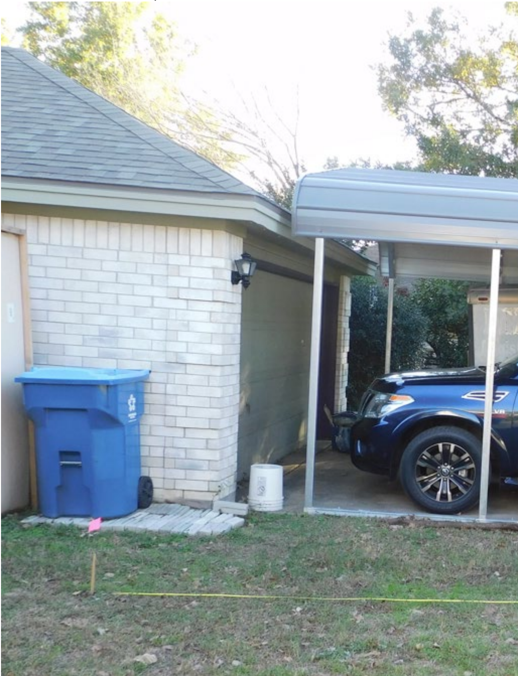
Photo #3 shows the proximity of the carport to the roof overhang of the house being 6 inches.
