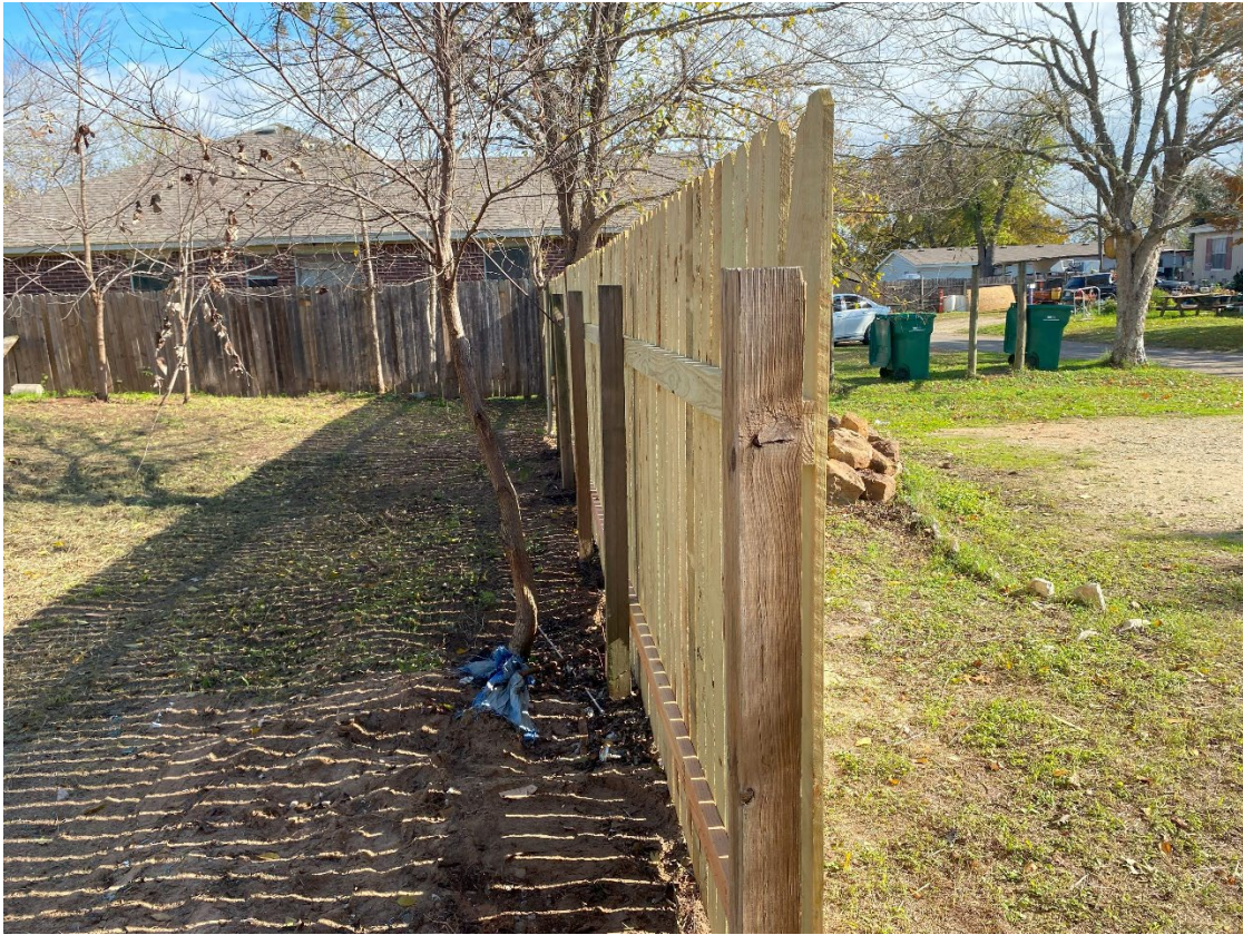
Both the rails and the pickets were replaced in this section of the fence (front east side).
